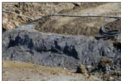
The first layer of the stabilised silt is reintroduced over the fly ash.
