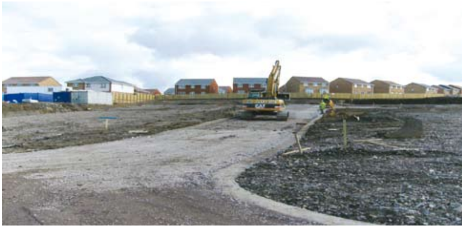
The new roads are supported by a rafted methodology over a deep silt layer
