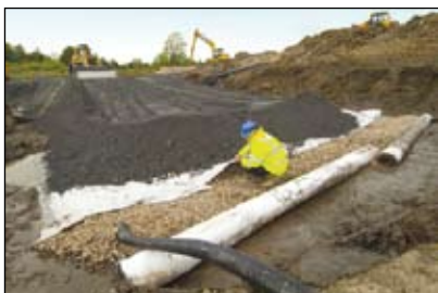
The fly ash is placed over the geotextile that overlays the stone and combined geotextile/geogrid layer.
