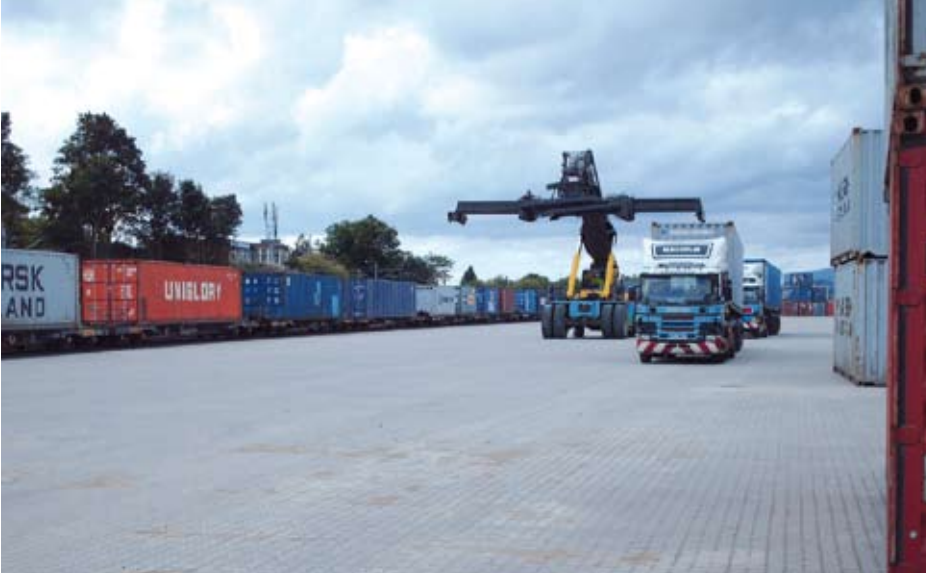
The new container handling facility withstands extremely heavy loads
