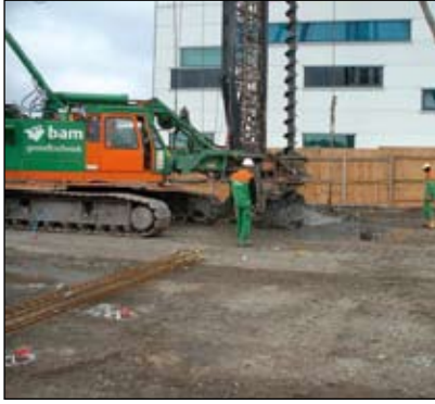
The completed stabilised platform with piling rig working on the cured and protected surface
